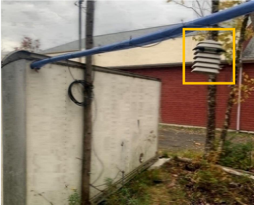
Figure 107 : External temperature sensor installed
