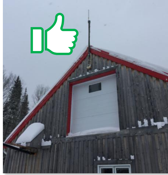
Figure 121 : Antenna on a building properly installed
